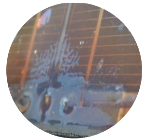
Delamination and corrosion 15 years Southern China
