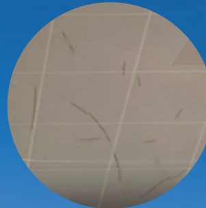
Widespread backsheet cracking PVDF
